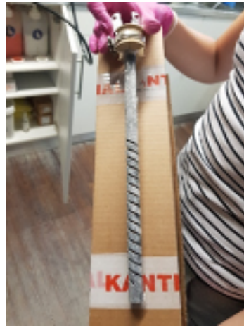
Fig. 2: SiC heating elements affected by deposits
